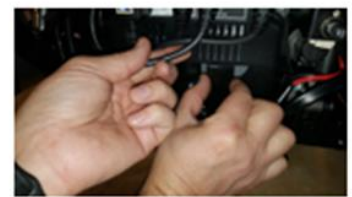
Pull out the wires in the power module
