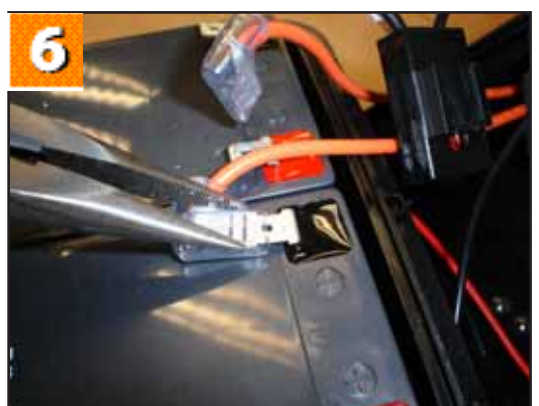
6. and the negative terminals on both batteries.
