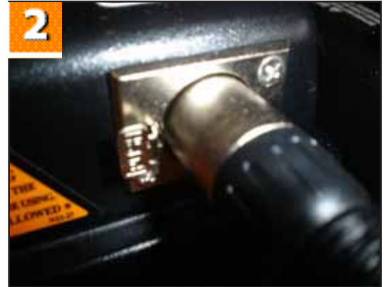
2. Shows the power lead connected to the battery.
